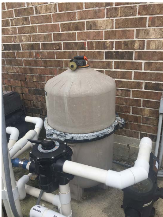
Fig. 3.21. A swimming pool filter that uses diatomaceous earth as a filter medium.
