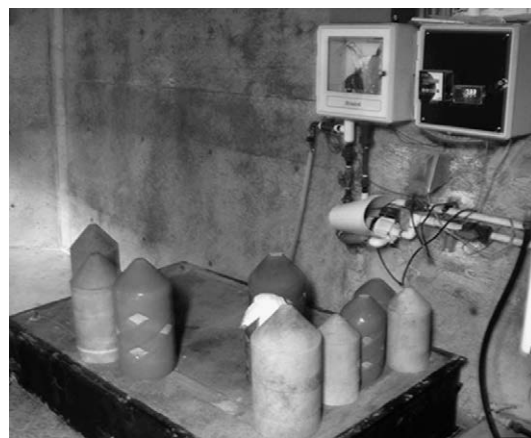
Fig. 3.41. A group of pigs of various sizes used to clear fouling organisms from pipes.
