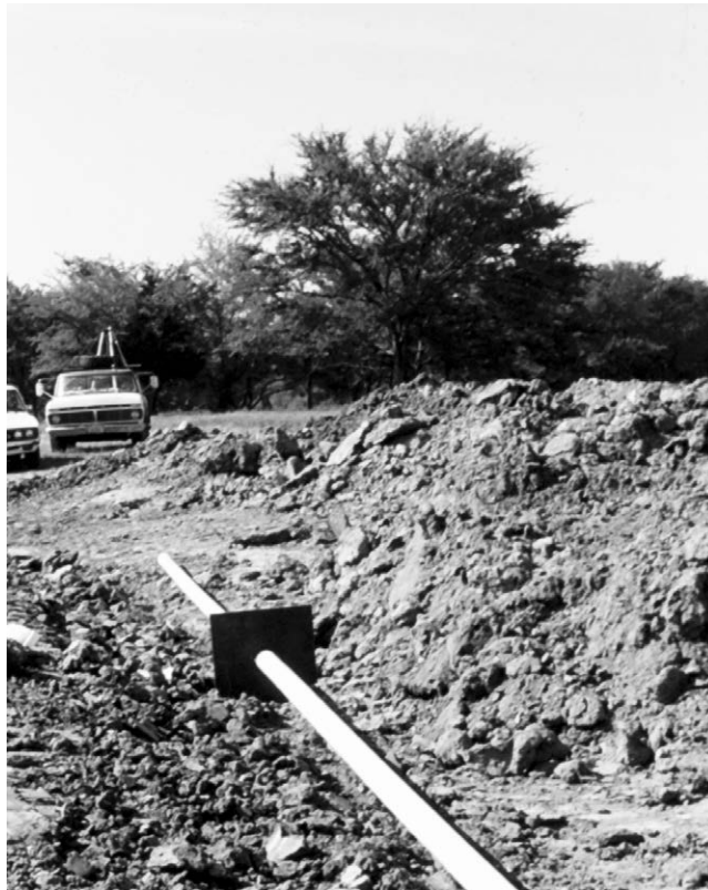
Fig. 3.9. A metal antiseep collar set in place immediately prior to having the levee built over it.
